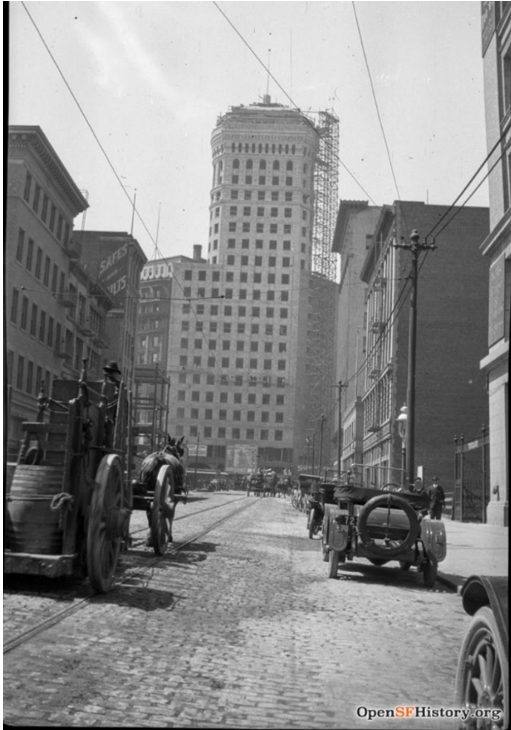
Figure 3 Hobart Building under construction, 1914, viewed from 2 nd Street, looking north toward Market Street; Source OpenSF History
